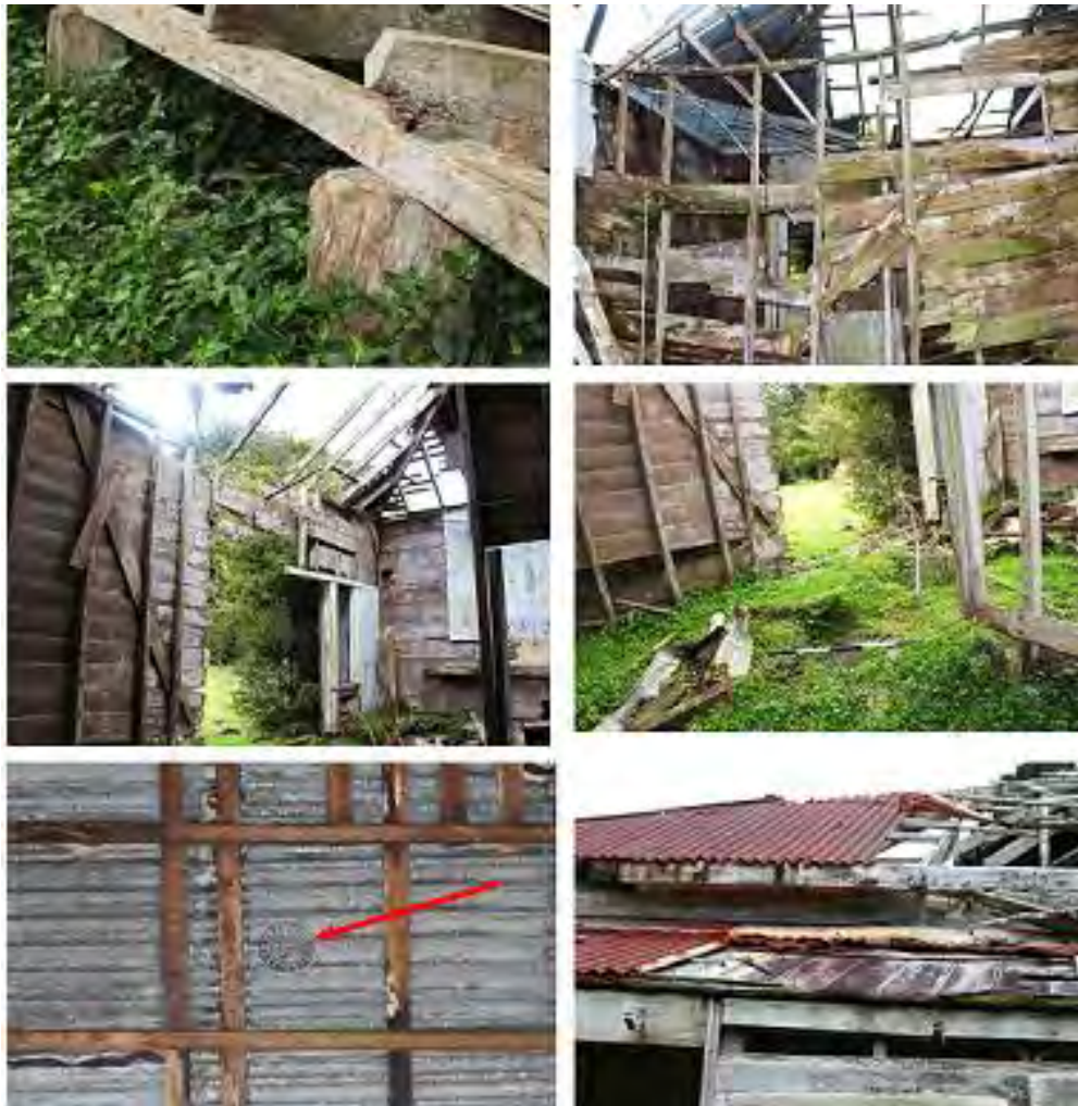
Figure 79 – Woodthorpe structure. Top (left) looking at piles/ subfloor and (right) looking at W-E cross-section through the house; Middle (left) looking at southern wall/ roof where chimney would have been and (right) looking at likely former location of a back to back fireplace; Bottom (left) stamped corrugated iron and (right) detail of roof construction for house and lean-to addition
