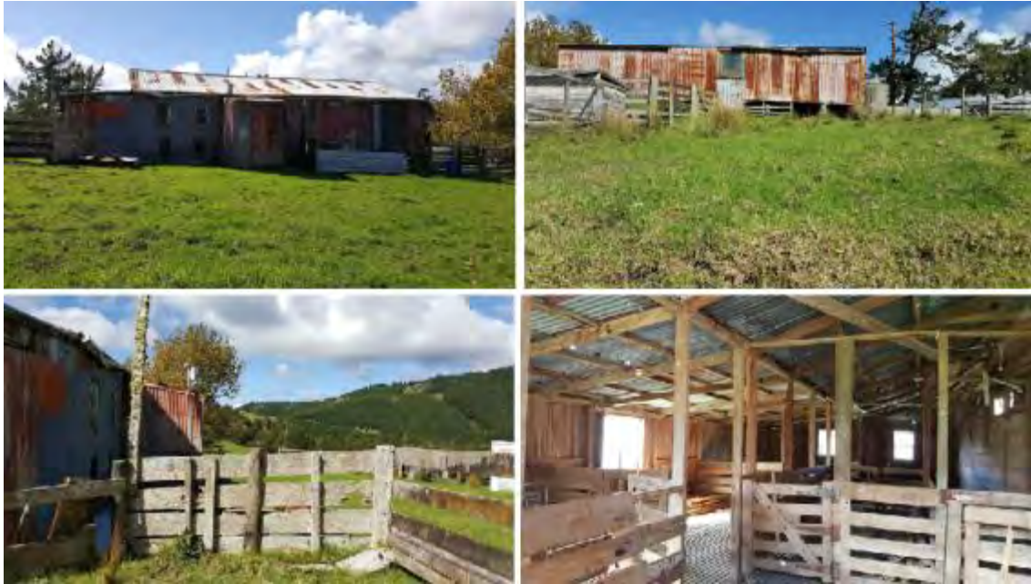
Figure 67 – Woolshed at 1207 SH1. From top – west facing elevation (left); east facing elevation (right); bottom – lean to extension and fencing on the west side of the shed (left); internal view of the shed (right)
